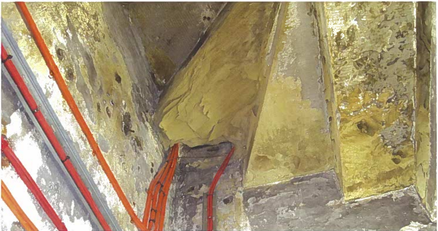
Photograph of the underside of the damaged tread showing extensive delamination and damage. It also shows the surface coating of the stone.
