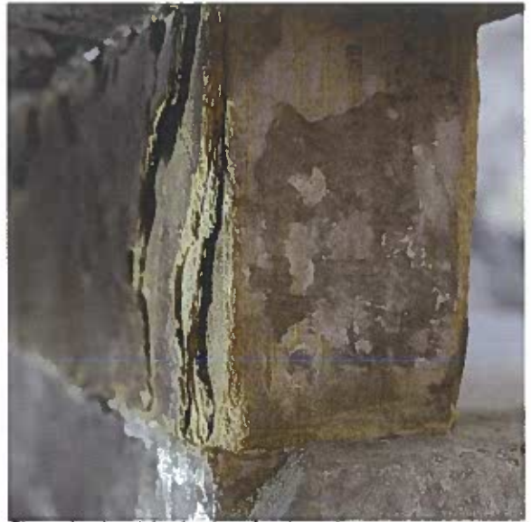
Photo showing delamination of a stone riser
