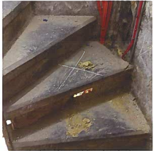
Photo showing damaged tread and riser to be replaced
