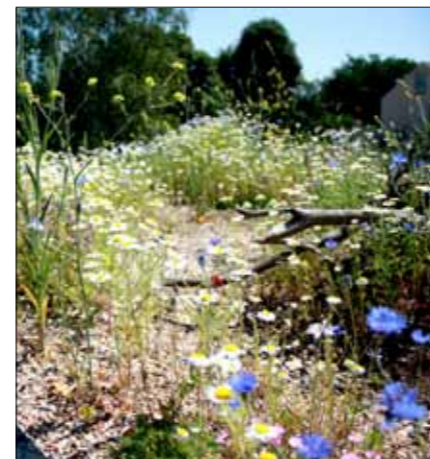
Extensive Green Roofs - Wildflowers/Biodiverse Roof
