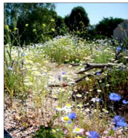
Extensive Green Roofs - Wildflowers/Biodiverse Roof
