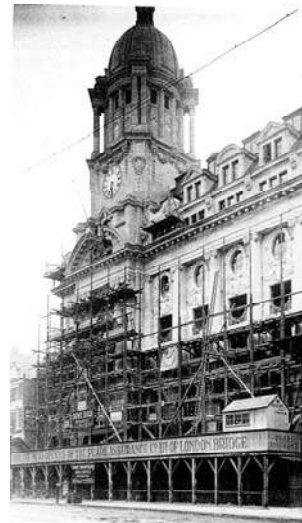
Wooden scaffold surrounding the High Holborn façade of the Phase I works 1913.
