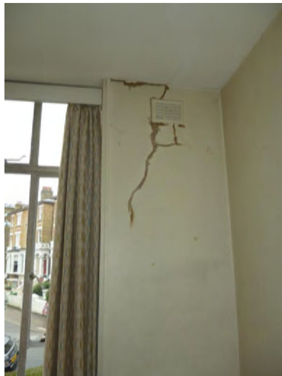
Figure 4: Internal cracking of the northern wall on the second floor.
