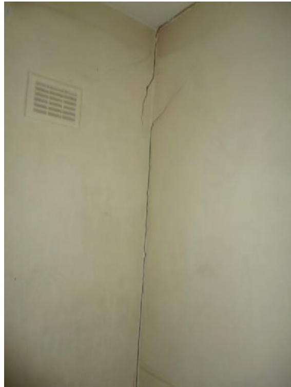
Figure 3: Internal cracking of the southern wall on the third floor
