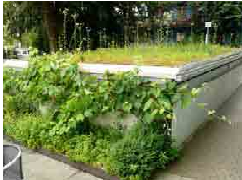
Biodiverse living roofs to garden store and heat exchanger unit
