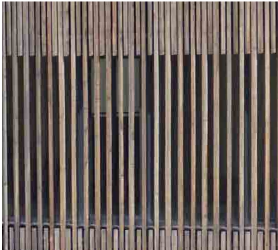
Vertical timber screen fencing is difficult to climb. Doors to heat exchanger/Garden store can be incorporated.
