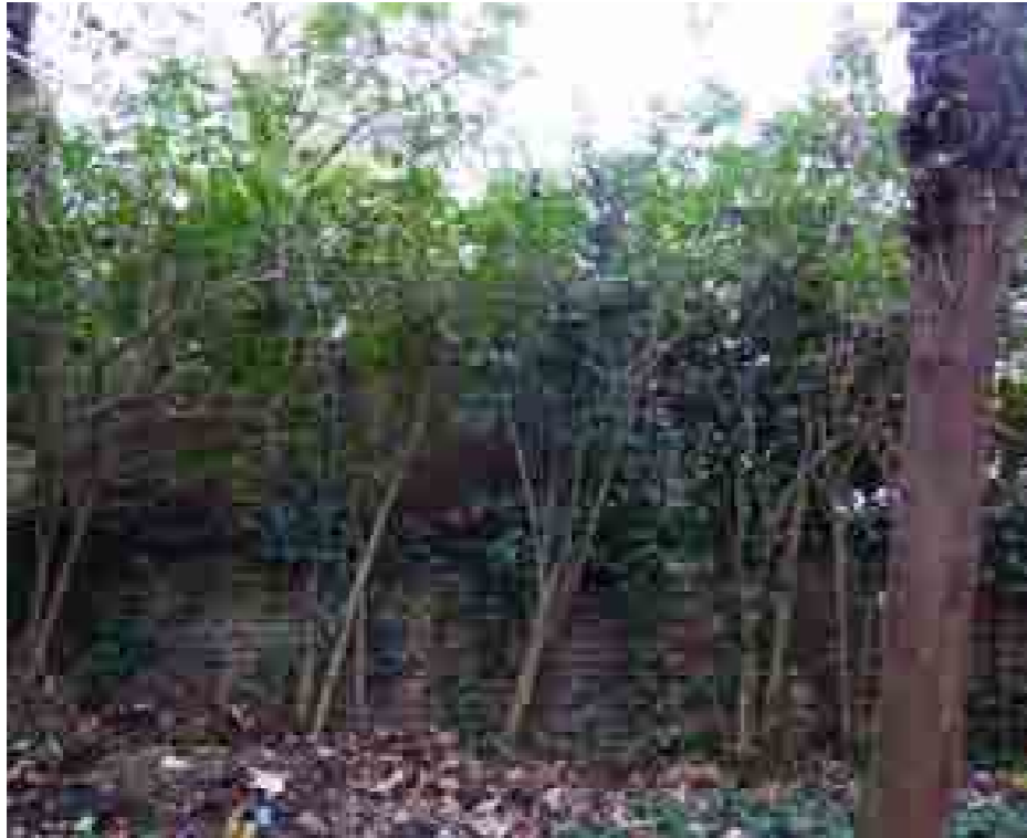
Overgrown privet hedge and brick walls to each side of rear garden
