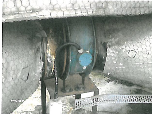
Non-asbestos vibration damper on ductwork on roof.
