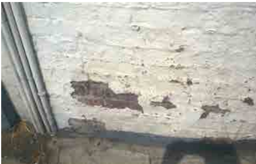
Photograph 2.8: Flaking paint on outside wall of the building
