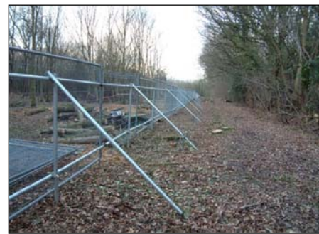
Photo 2: Heras fencing wired to scaffold braced posts is a robust and effective interpretation of the BS specification.
