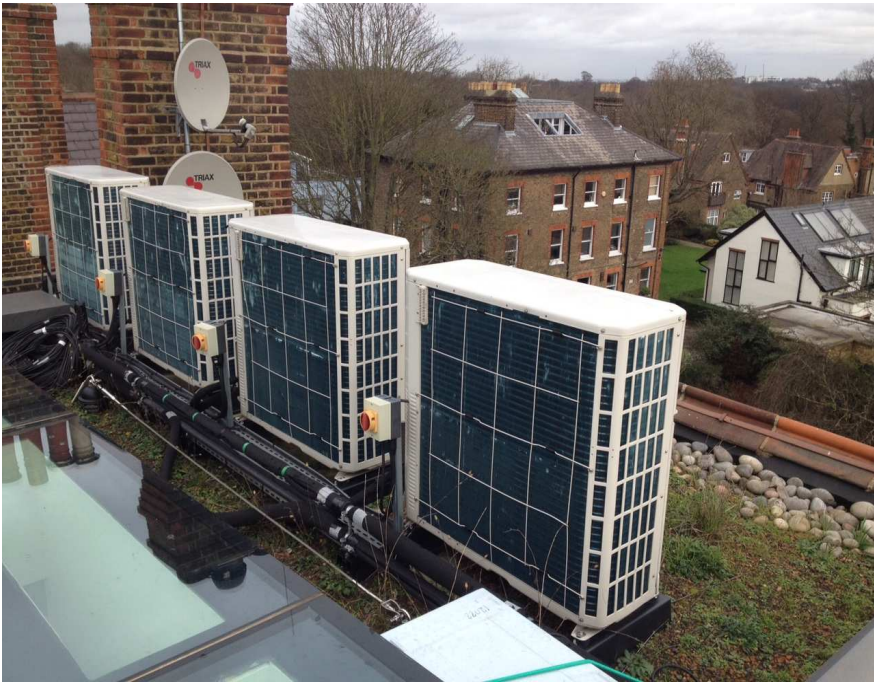
Air conditioning condensers
