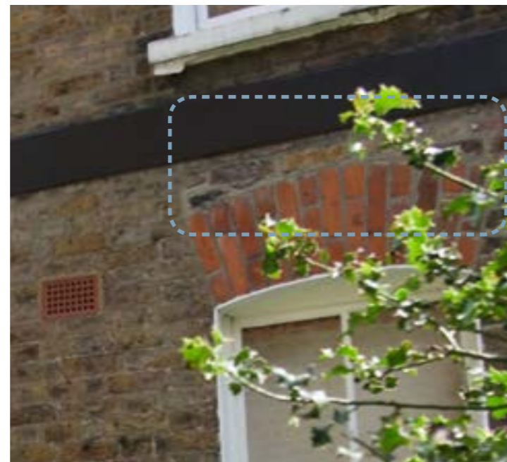
3. Infill brickwork to previous main entrance along the South West elevation clearly visible above the window arch as seen with the differing colour bricks and paler pointing.
