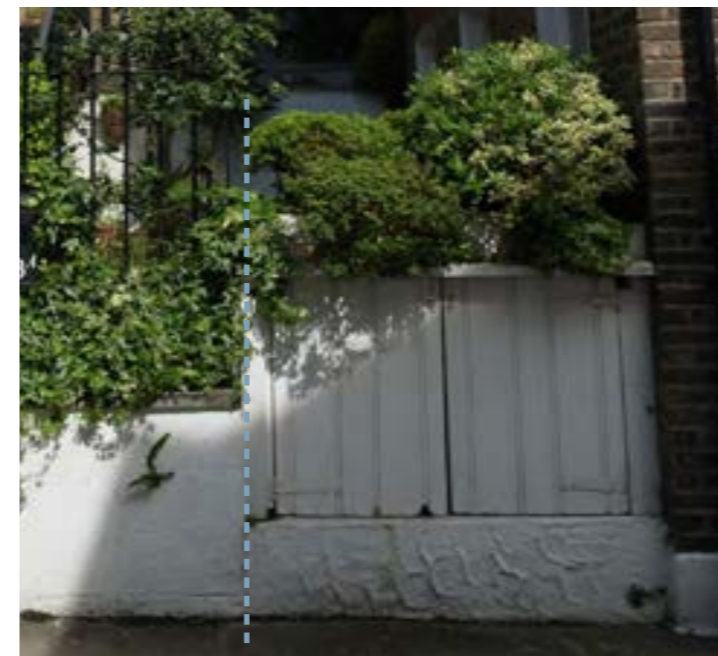
4. Original location of off street entrance visible as indicated by the blue line, the change in masonry styles, and the lack of original features such as coping stone and railings.
