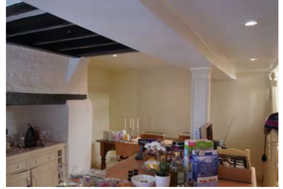
3. Low and inconsistent ceiling levels at Lower Ground Floor likely resulting from changes to the floor level above over the years.
