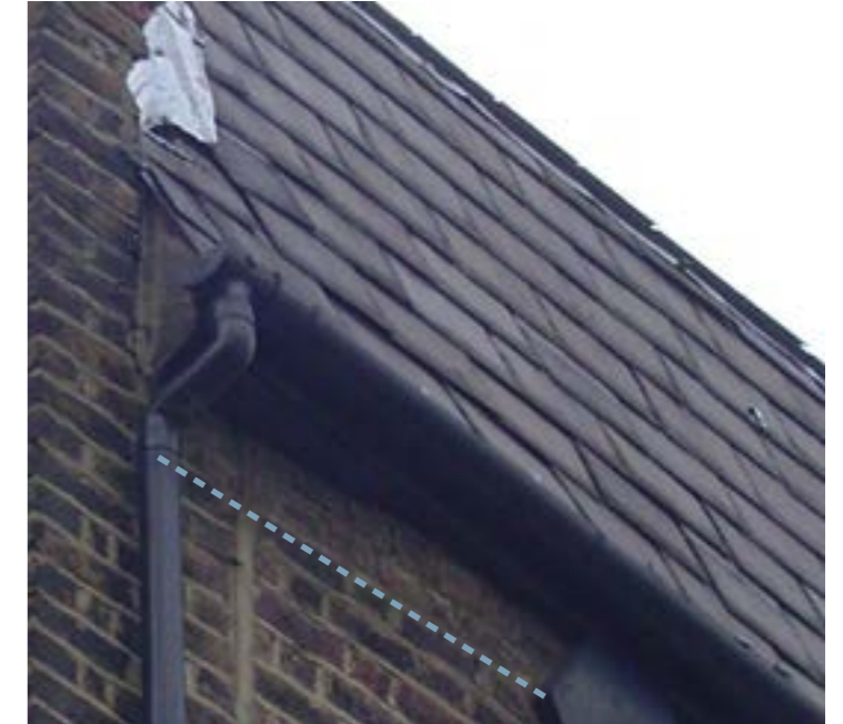
2. Mismatching colours of the upper two brick courses indicate the extent to which we suspect the old parapet was removed when the loft extension was introduced.
