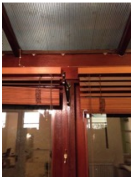
Existing Timber Framed Sliding Door and honeycomb polycarbonate sheets between the timbers.
