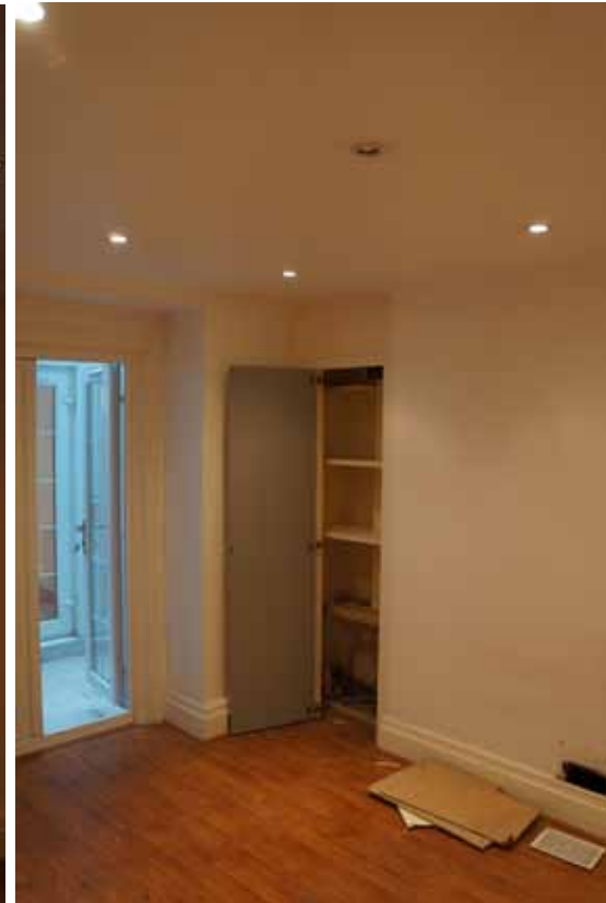
B6. SERVICES AND MISSING FIREPLACE
