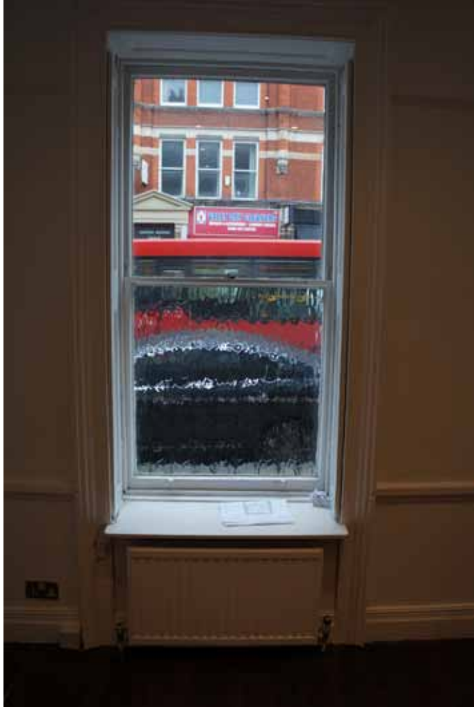
G7.NON-ORIGINAL SASH WINDOW WITH MISSING GLAZING BARS
