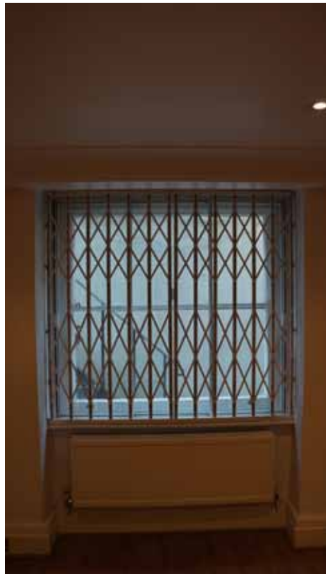
B5. NON-ORIGINAL TIMBER SASH WINDOW
