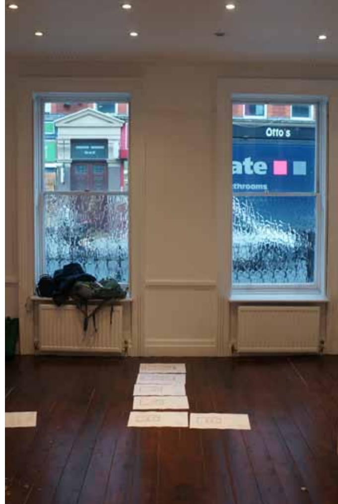
G8.NON-ORIGINAL SASH WINDOWS IN POOR CONDITION FACING FRONT OF PROPERTY
