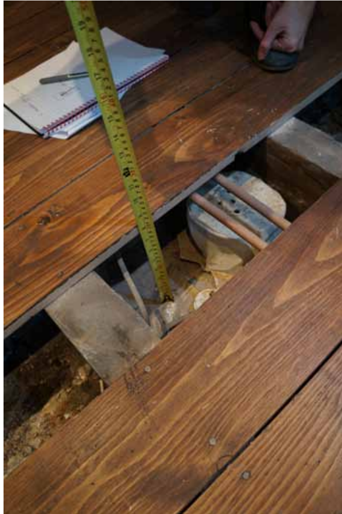
T3. NON-ORIGINAL FLOOR BOARDS
