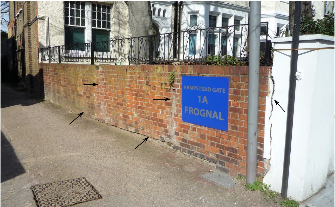
View along the side wall showing horizontal and vertical cracking and the corner pier detaching and leaning towards the pavement. Trunk of the beech is behind the wall about half way along and the smaller lime is behind the pier and metal post.
