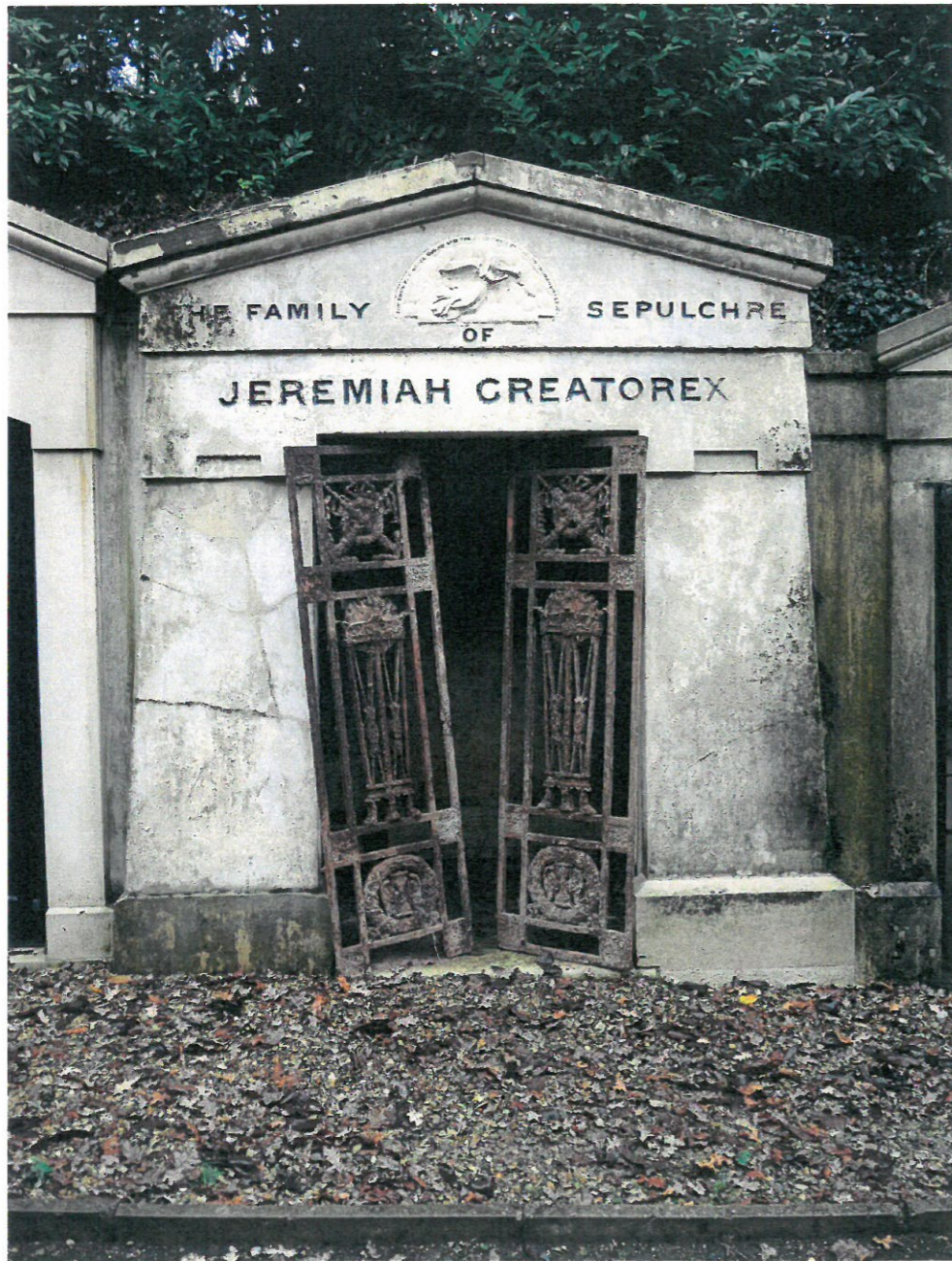
GRETOREX: LOST DOORS TO BE REFURBISHED & REINSTATED
