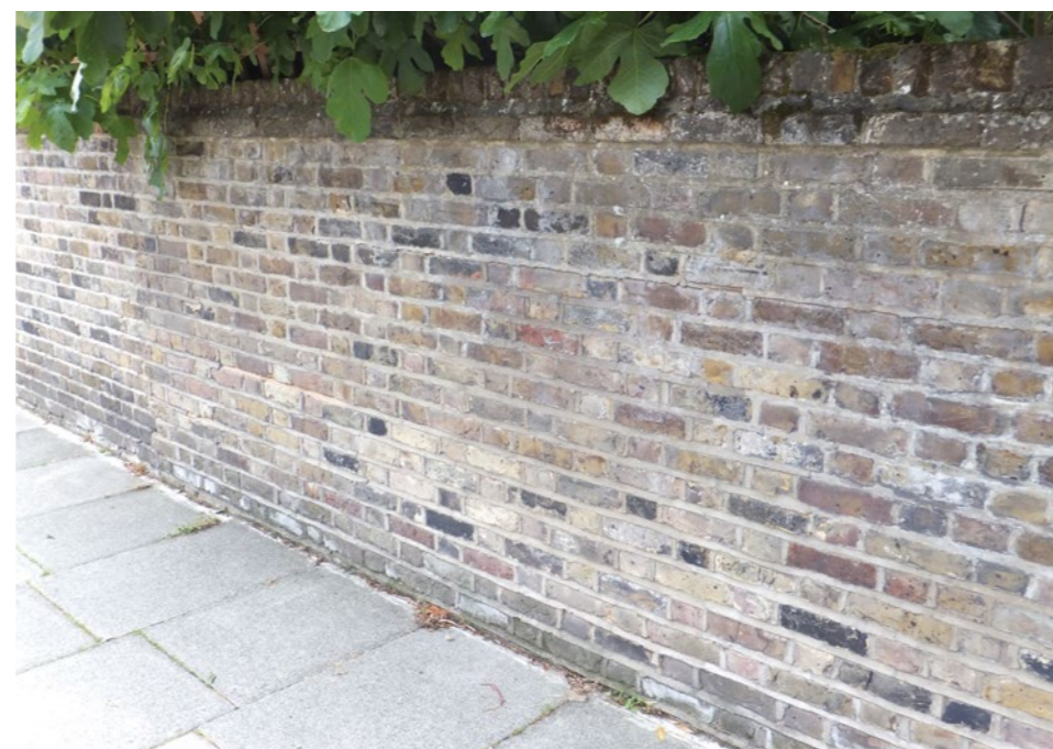
Garden wall, York Rise The most common local material is a light coloured Gault clay London stock brick.
