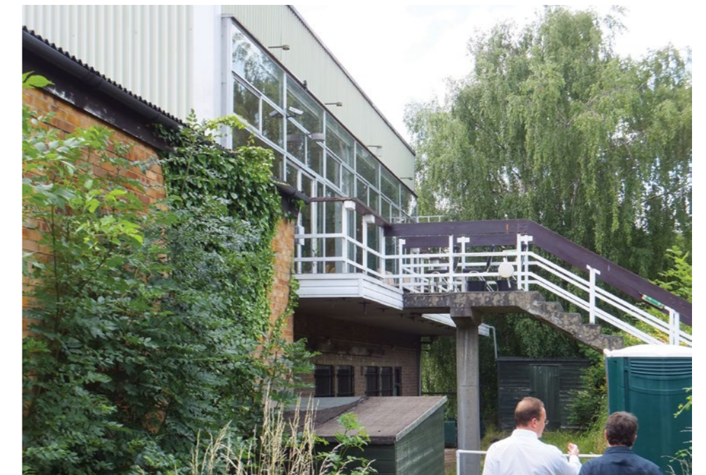
Northern elevation of Clubhouse A second bar on the first floor of the clubhouse looks north with generous views over the external bowling green and tennis courts in the northern part of the site.
