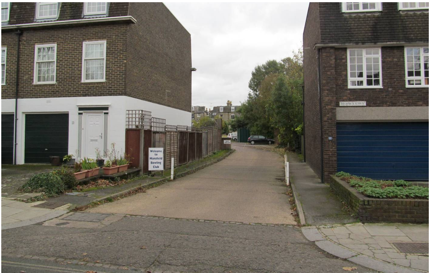
Photo 1 Existing 4.7m access road and 1.3m pavement between town houses on Croftdown Road Note 1 Cracked paving with vehicles cutting corner to western channel [right hand side]
