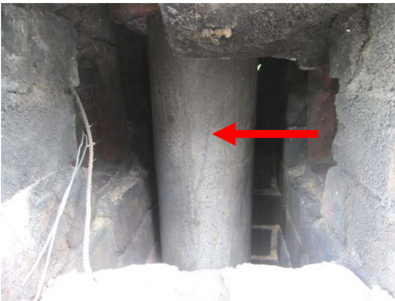
Visual inspection - Flue pipe to chimney - flat roof - Chrysotile (white asbestos) presumed. Full extent unknown.
