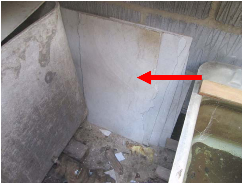
Sample 03 – Panelling & associated debris – water tank housing – Amosite (brown asbestos) & Chrysotile (white asbestos) detected.
