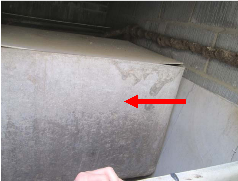
Visual inspection – 2x Water tanks – water tank housing – Chrysotile (white asbestos) presumed.
