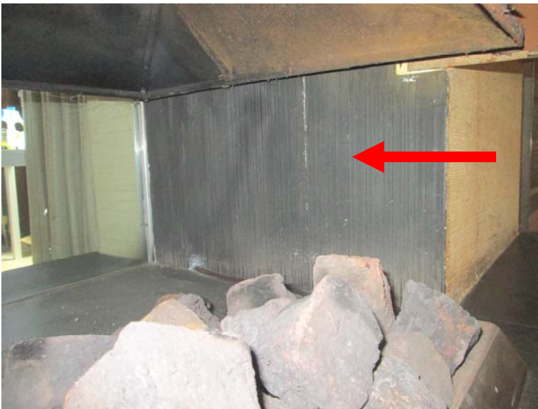
Sample 04 – Panels to fire place – lounge – Chrysotile (white asbestos) detected.
