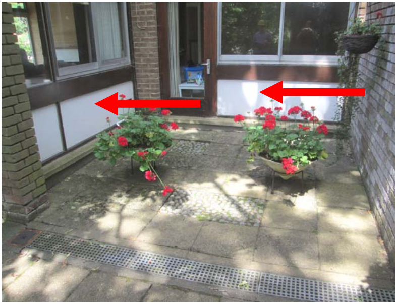
Sample 07 – Lower panels to side wall – external – Chrysotile (white asbestos) detected.
