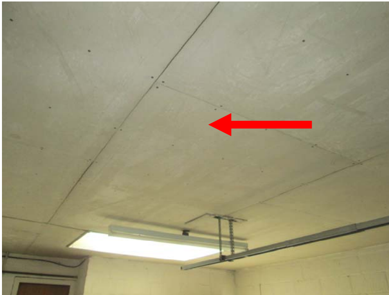
Sample 05 – Panels to ceiling – garage – Amosite (brown asbestos) & Chrysotile (white asbestos) detected.
