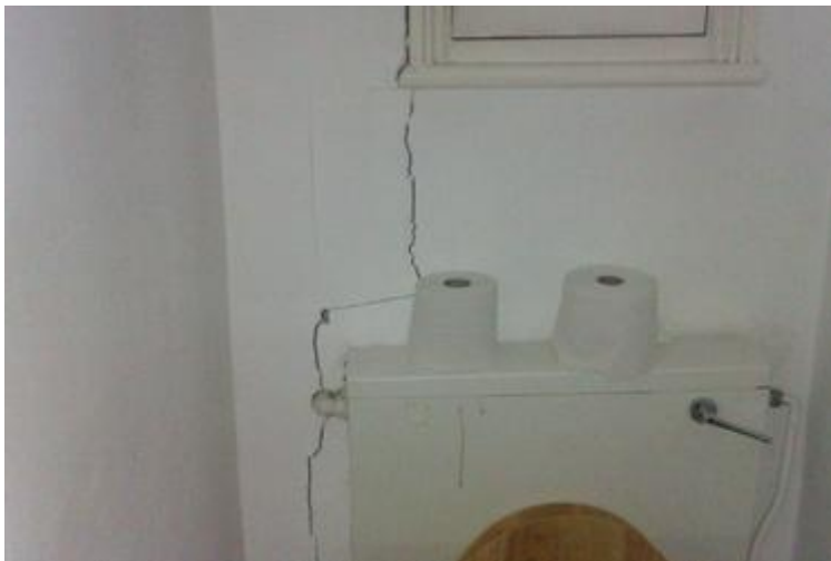
FIGURE 03 Tapered cracking recorded to ground floor toilet
