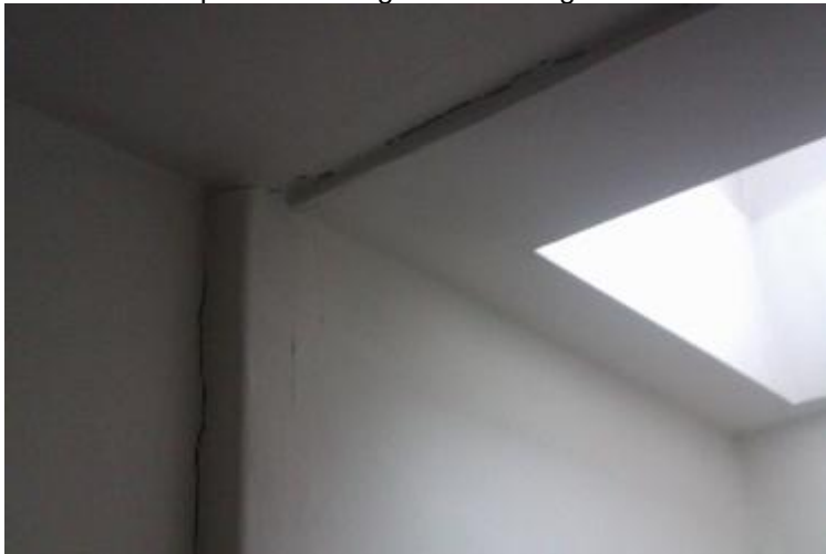
FIGURE 04 Horizontal and vertical cracking recorded at abutment to main frame house
