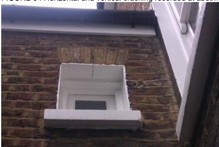
FIGURE 05 Cracking recorded above and below toilet window
