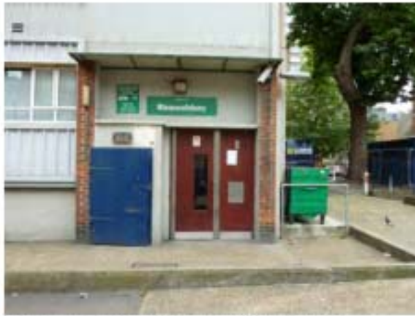
4- Entrance from Orde Hall Street adjacent to further external waste storage. Approach is blocked by kerb and level change.
