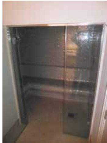
B9 Steam Room
