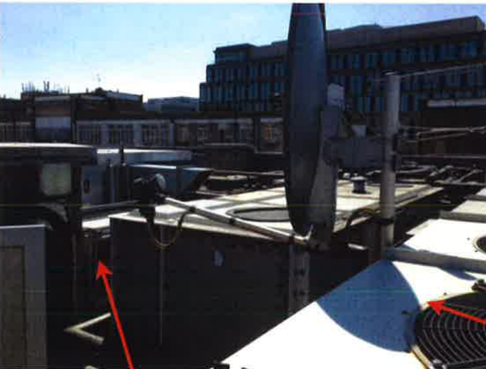
air handling unit vent out
