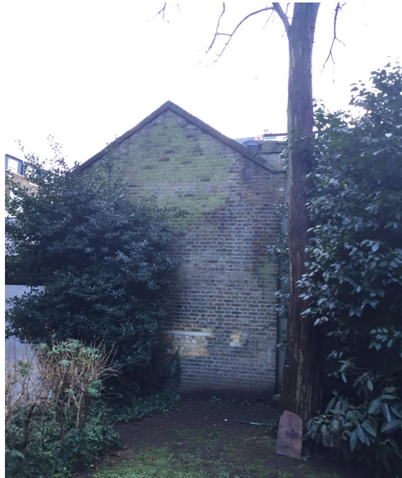
Photo taken from garden of No. 1A Primrose Gardens looking south-east towards the rear face brick elevation of No. 17 Elizabeth Mews.
