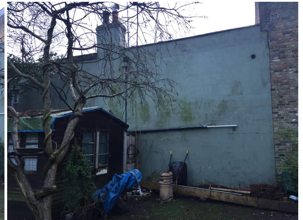
Photo looking south-east towards the rear elevation of No. 16 Elizabeth Mews. The proposed window is to be located beneath the horizontal drainage pipe (to be removed). The rear face brick elevation of No. 17 Elizabeth Mews can be seen to the right hand side of the image.
