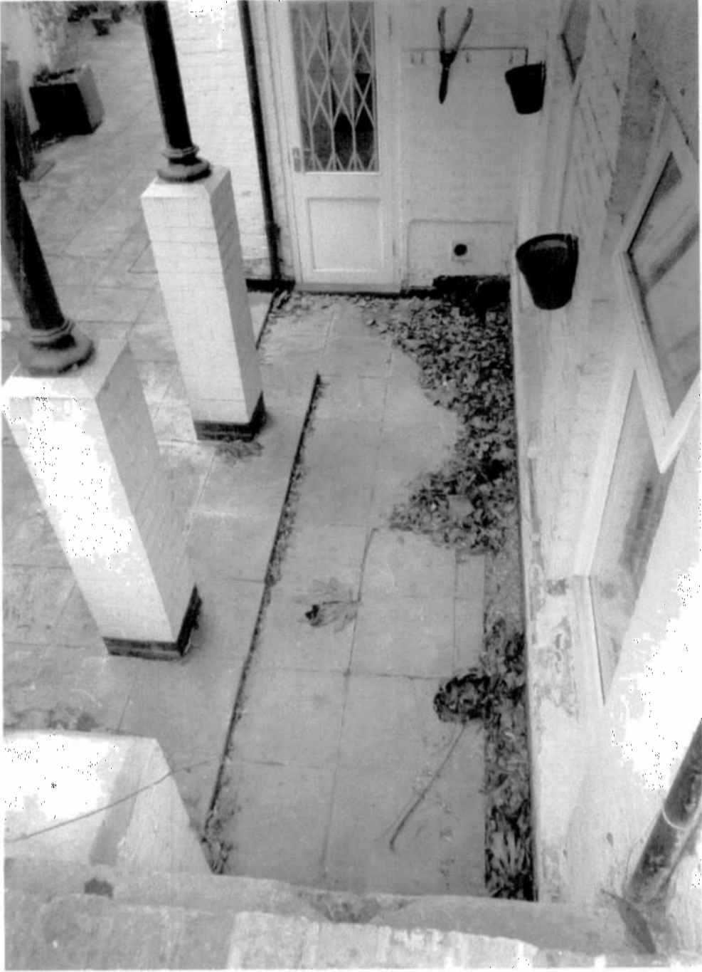
2015/0565/P SITE OF PROPOSED EXTENSION 64A FITZJOHN'S AVENUE SHOWING POSITION OF WASTE WATER AND RAIN WATER DRAINS
