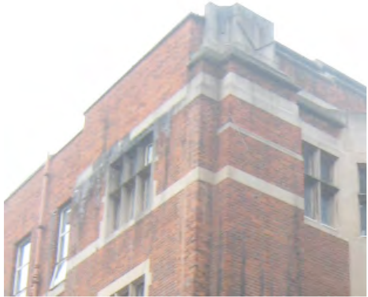
Figure 11: the altered parapets
