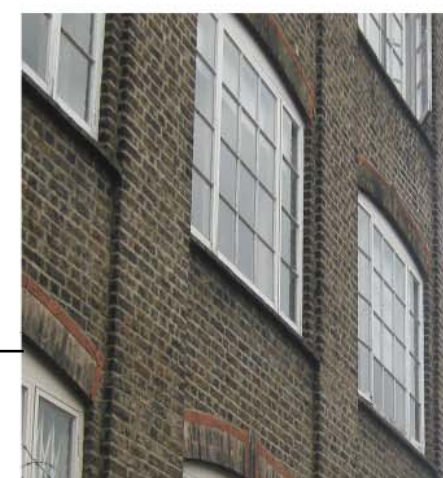
Existing bricks and reclaimed bricks to match. New windows to match existing
