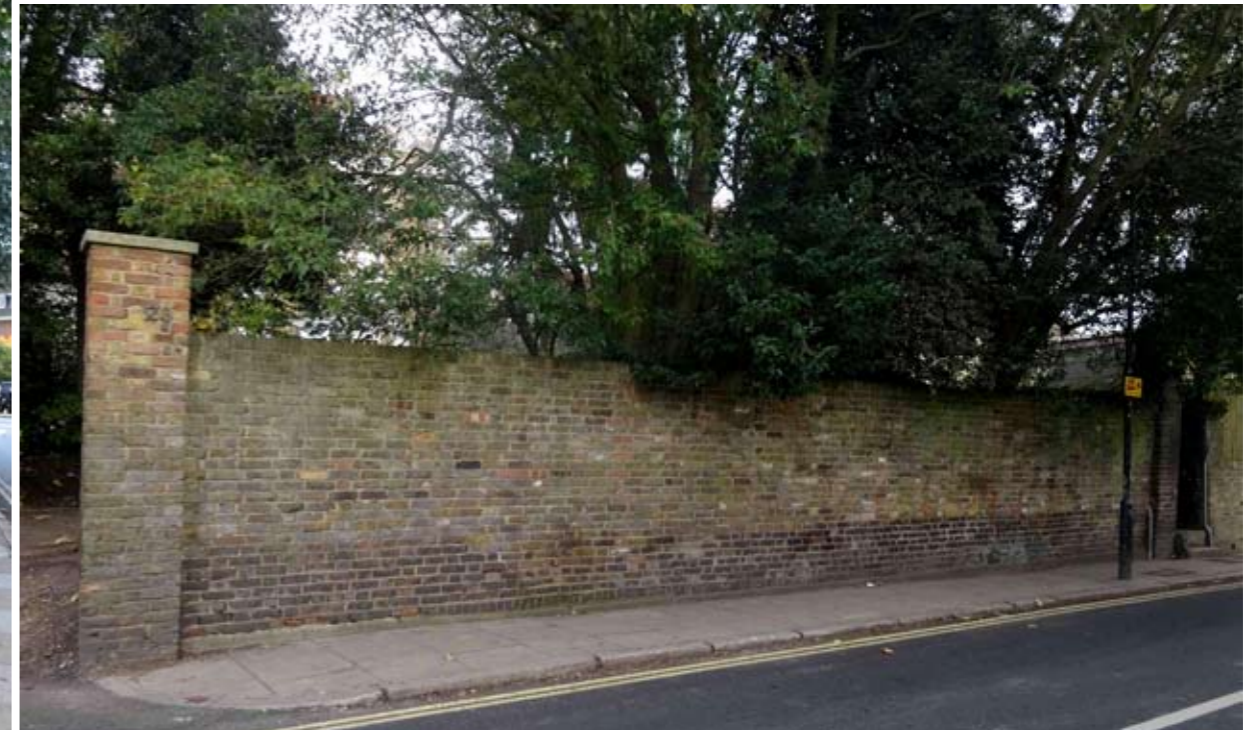
VIEW ALONG DEFECTIVE BOUNDARY WALL FROM FROGNAL LANE SHOWING BANDING OF EARLIER BRICK TO THE LOWER COURSES
