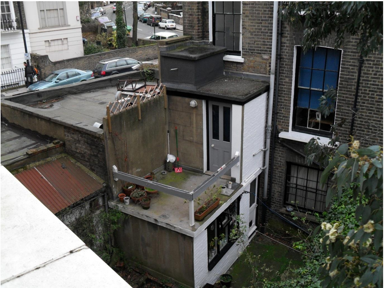
5.11 Rear view of No 46 Inverness Street over the rear garden of No 24 Gloucester Crescent
