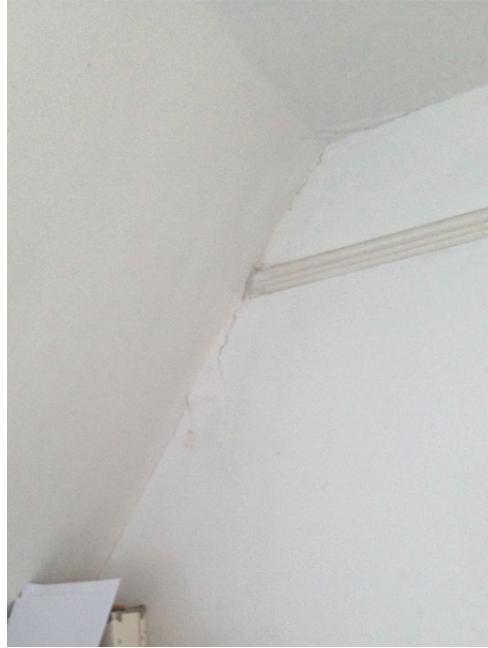
Figure 4 Crack 1 - 2nd floor
