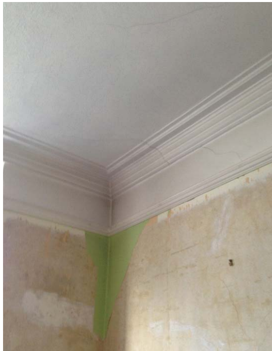
Figure 5 Crack 2 first floor
