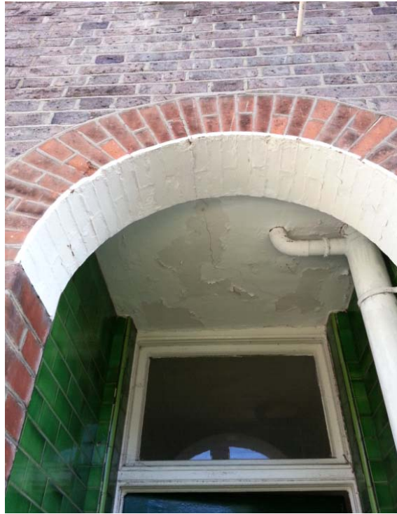
Figure 6 Crack 3 front elevation
