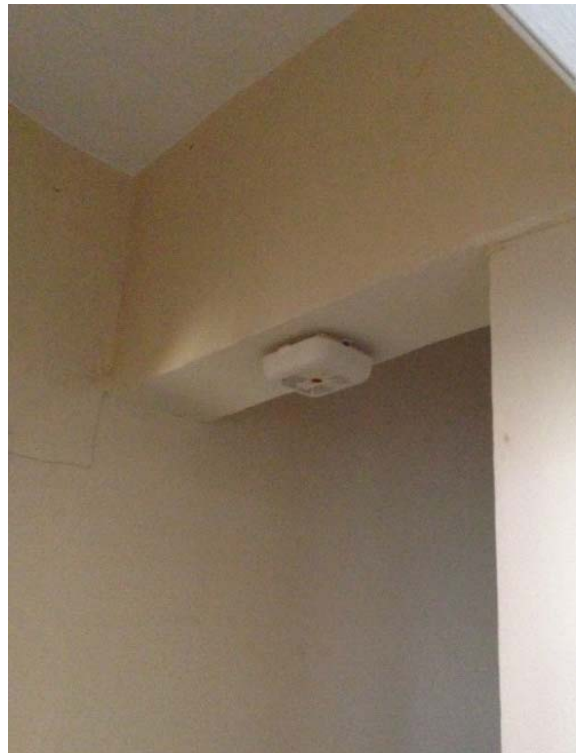
Figure 7 Crack 4 - below the beam
