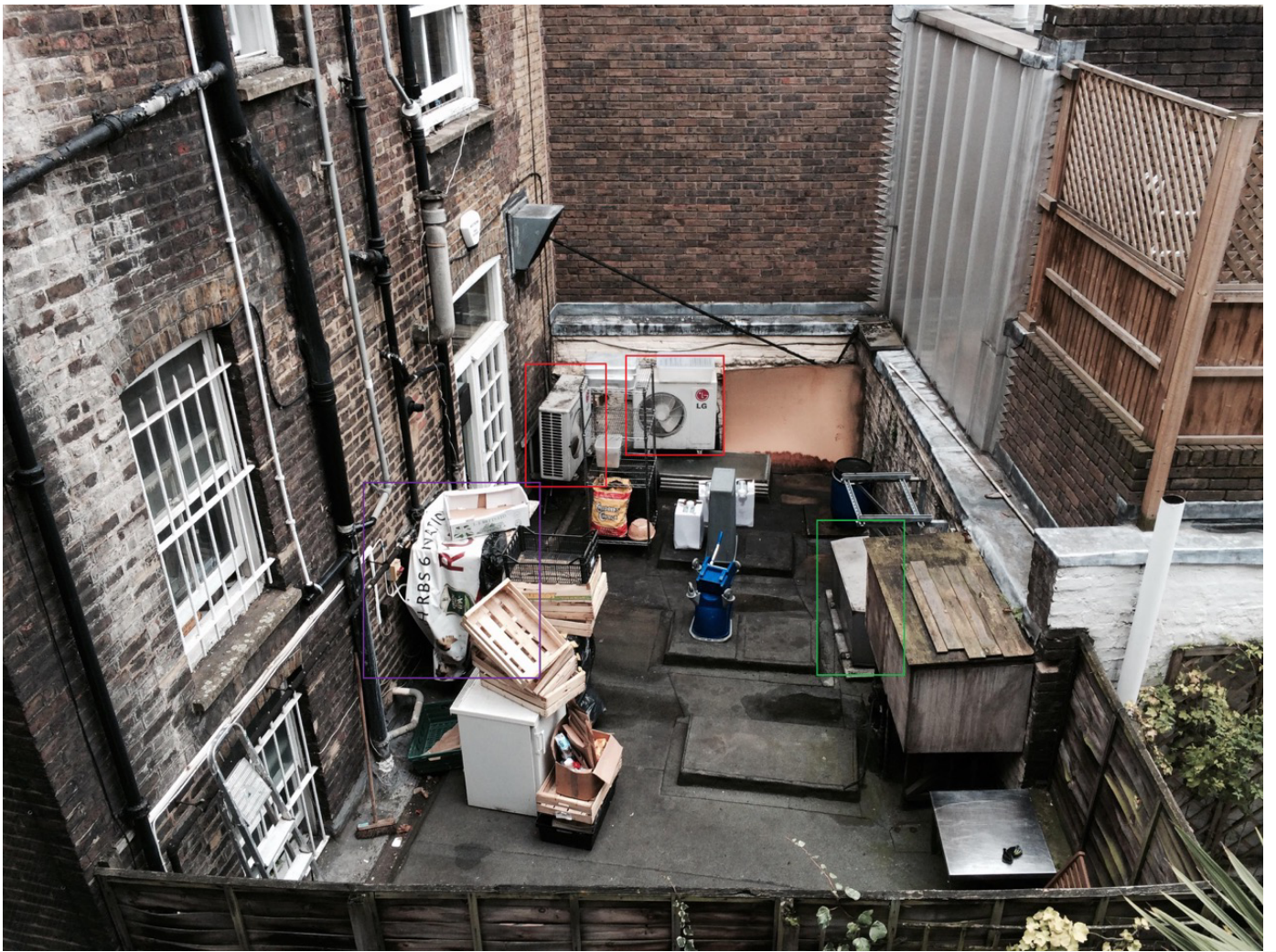
View of first floor roof and rear elevation of 28 Warren Street (from 20 Conway Street)
