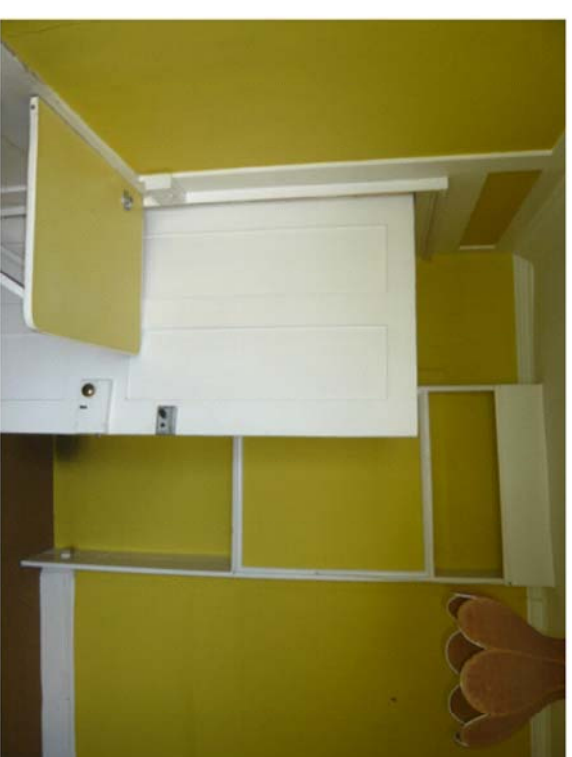
Strip and repaint timber door. Retain skirting and architrave. Retain and repair cornice.
