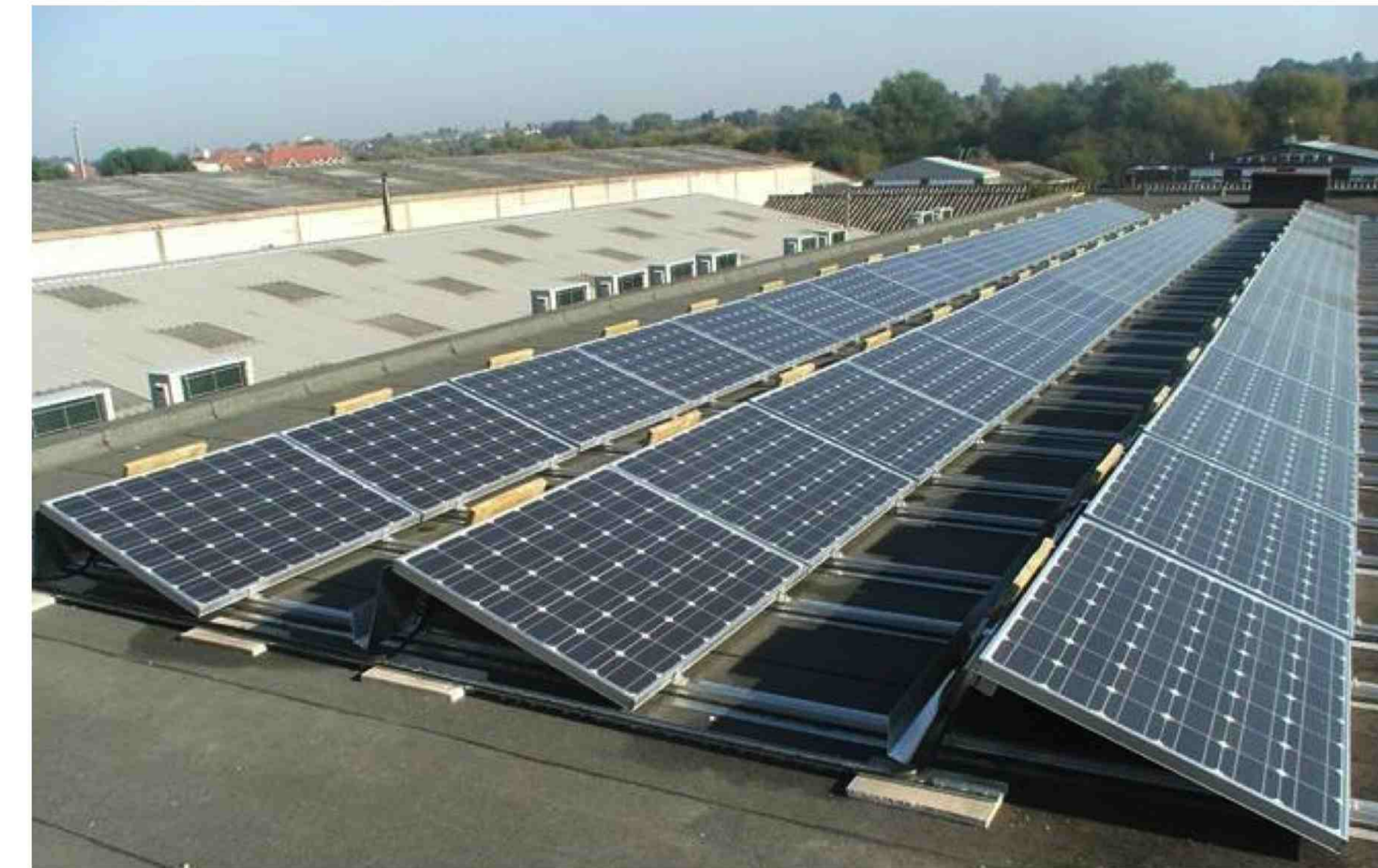
SOLAR PHOTOVOLTAIC PANELS ON LOW PROFILE, BALLASTED MOUNTING SYSTEM
