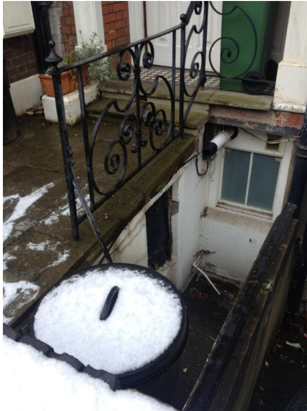
Photo 1- Existing lower ground window to be replaced with timber framed obscure glazed door
