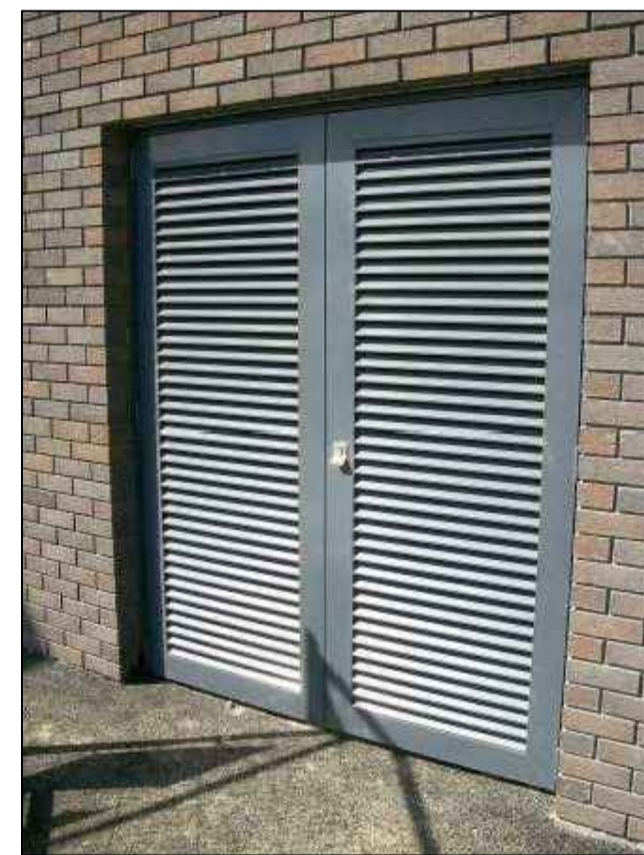
IMAGE REFERENCE FOR EXTERNAL DOOR / IRONMONGERY SPEC TO COMPLY WITH BUILDING CONTROL
