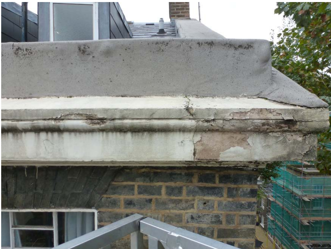
Photo 22: Taviton Annex - asphalt over parapet.
