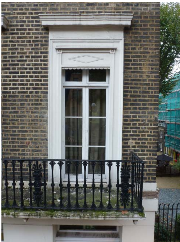
Photo 29: Taviton Annex - balcony doors.
