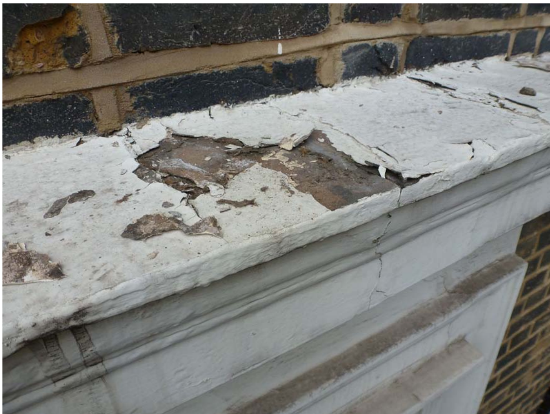
Photo 28: Taviton Annex - window surround.
