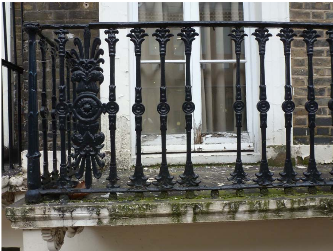
Photo 31: Taviton Annex - balcony railings - typical defects.
