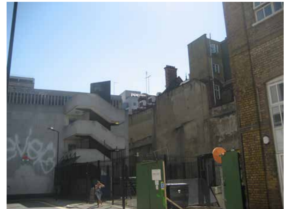
Fig. 4.25: Rear side of 9-13 Grape Street faces a yard on West Central Street, sans any door or window openings.
