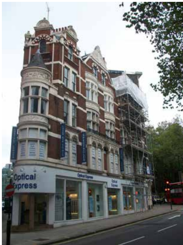
Fig. 8.5: (No. 4) 219 - 229 Shaftesbury Avenue is near to but not affected by the changes proposed to 9-13 Grape Street.
