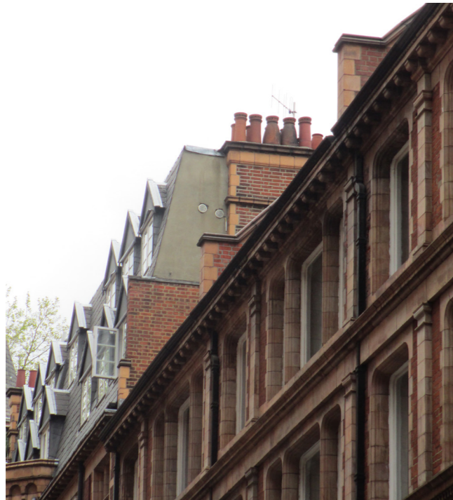
▲ 5: The south facing gable end of the mansard extension to Queen Alexandra Mansions
