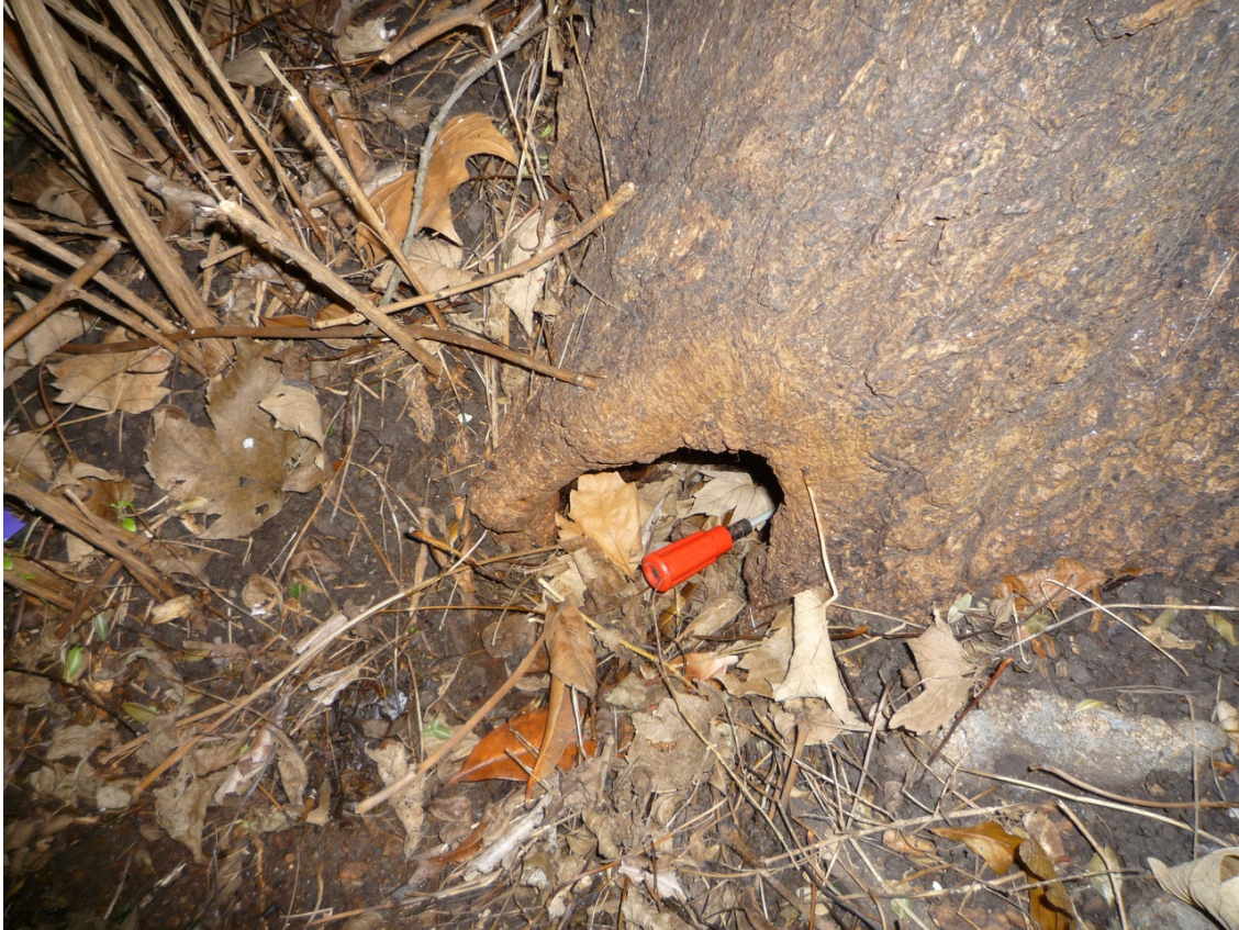
Probe inserted into the cavity on the SW side of the tree.
