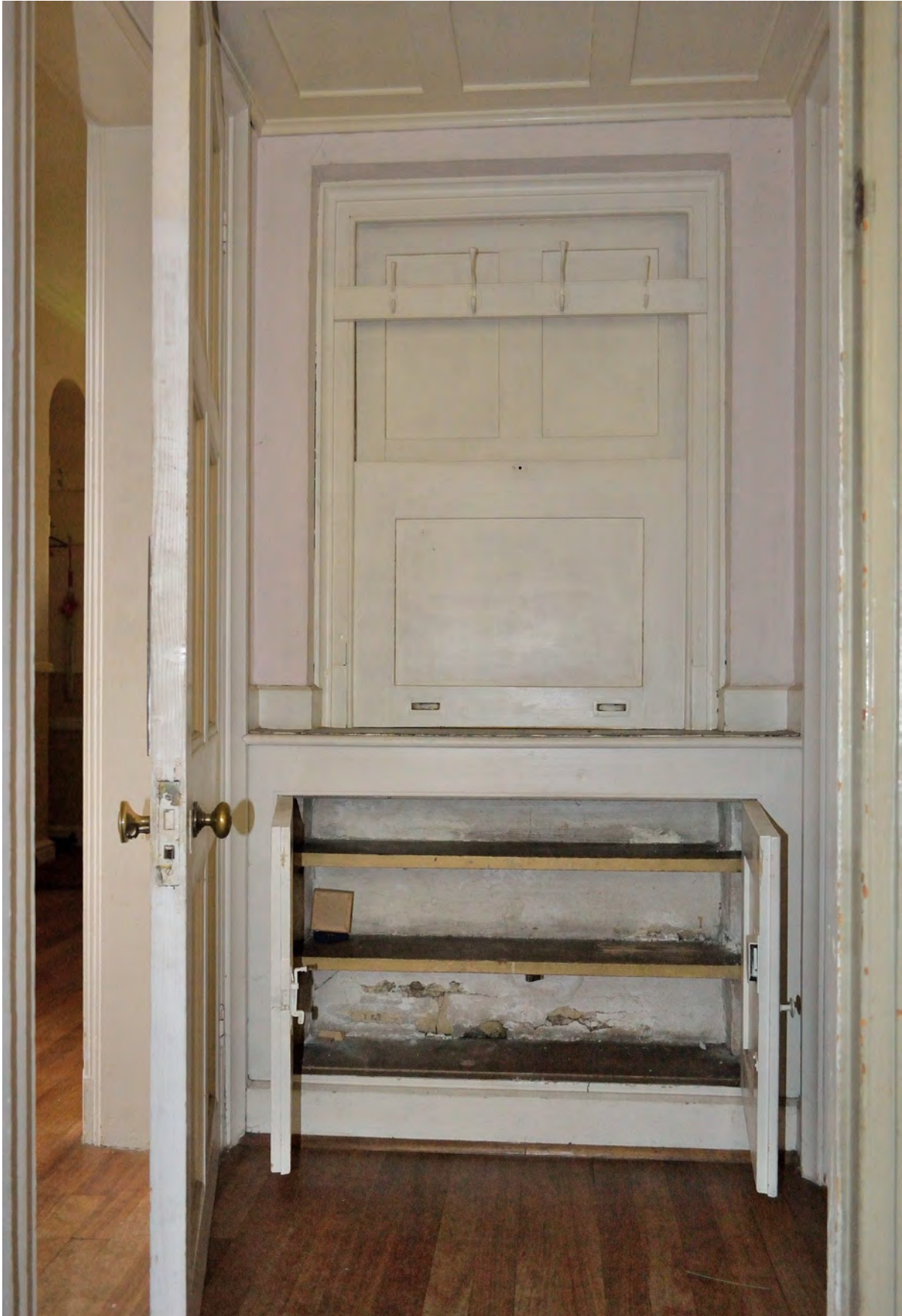
Fig 35, The kitchen / pantry lobby showing the closed serving hatch above a cupboard unit, which appears to be a historic detail. The wall behind also appears not to have been disturbed, and the skirting runs through.
