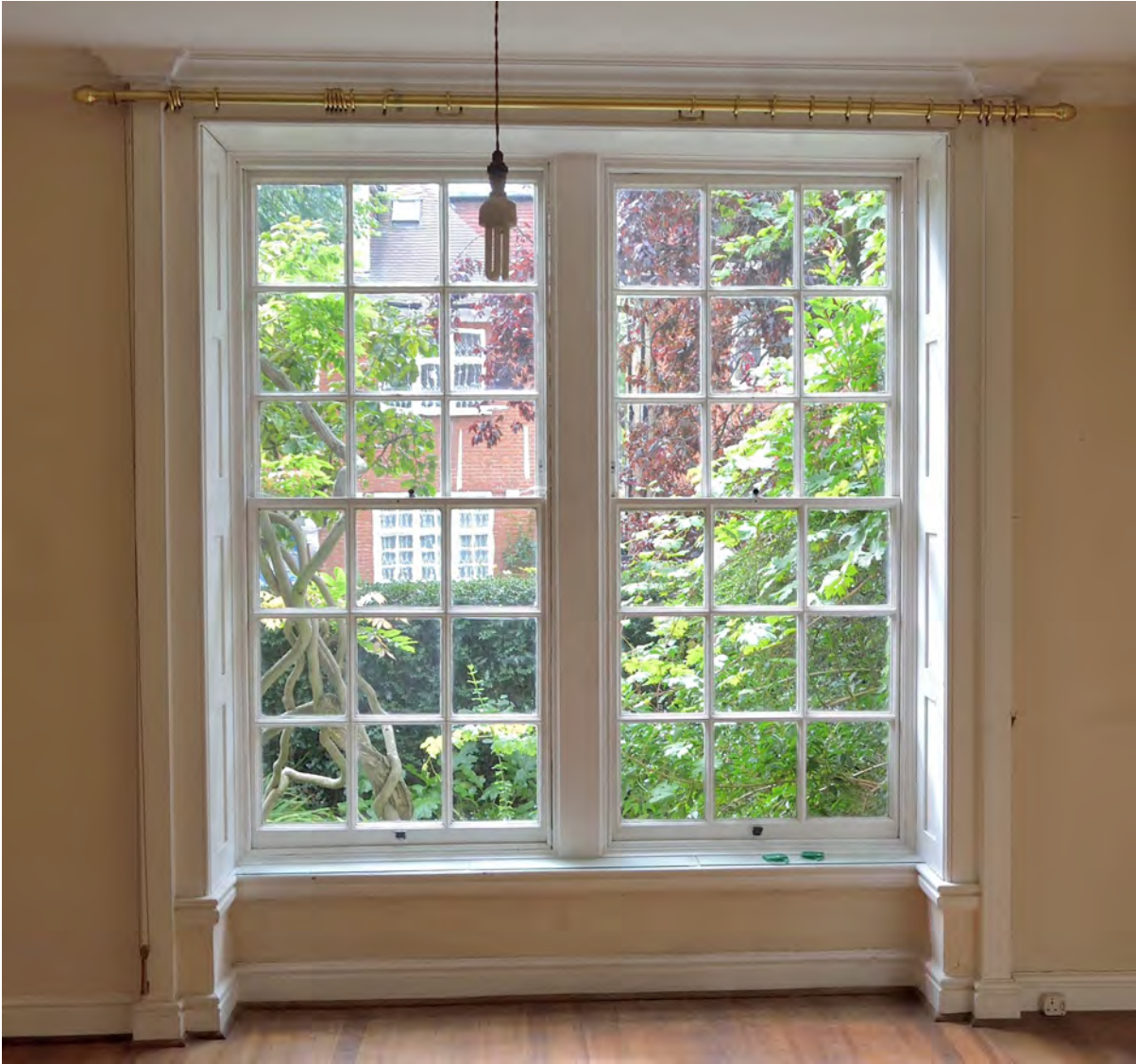
Fig 18, The original deep double sash window surviving in the dining room, with projecting architraves with pronounced moulded capitals and bases.
