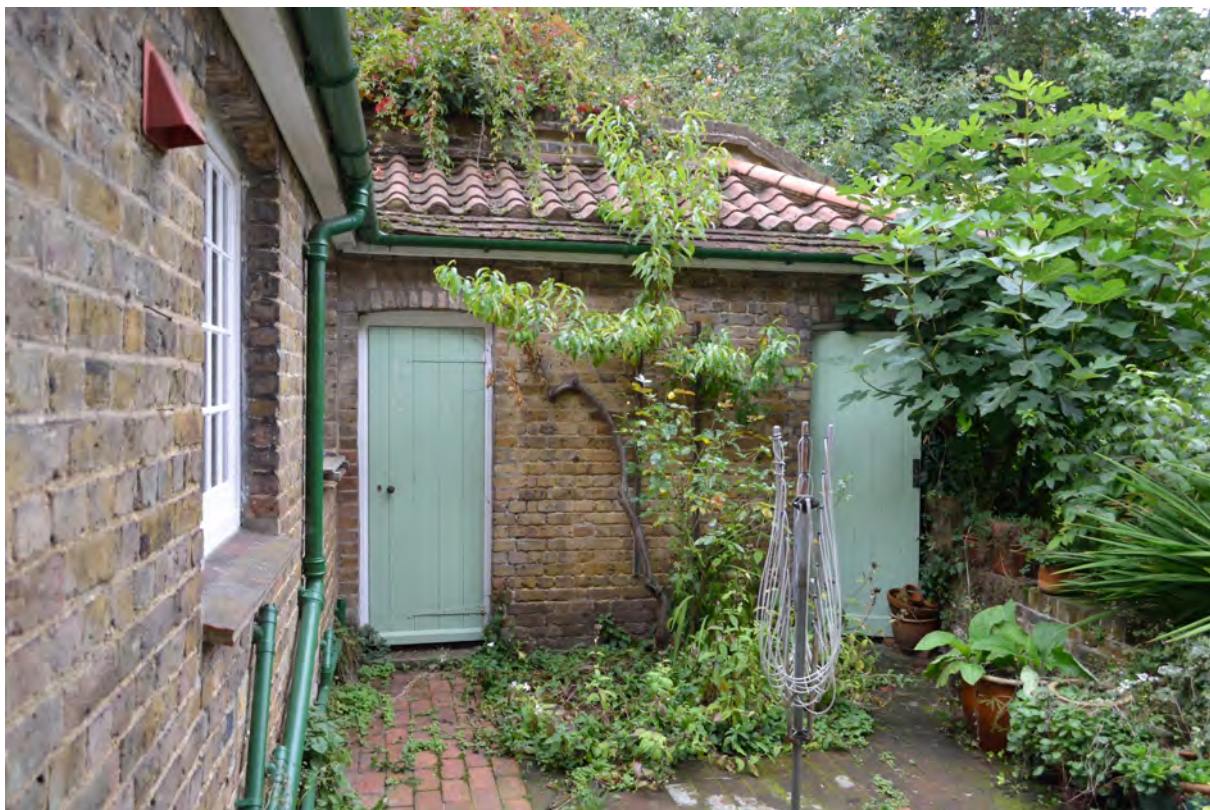
Fig 10. The end of the service range containing fuel stores within the small brick lined yard. The rounded tile hips to the roof are modern. .
