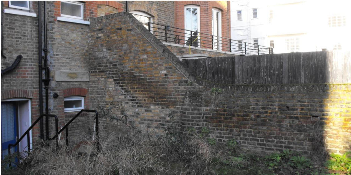
Figure 1: Sections A&B, damp patches visible
