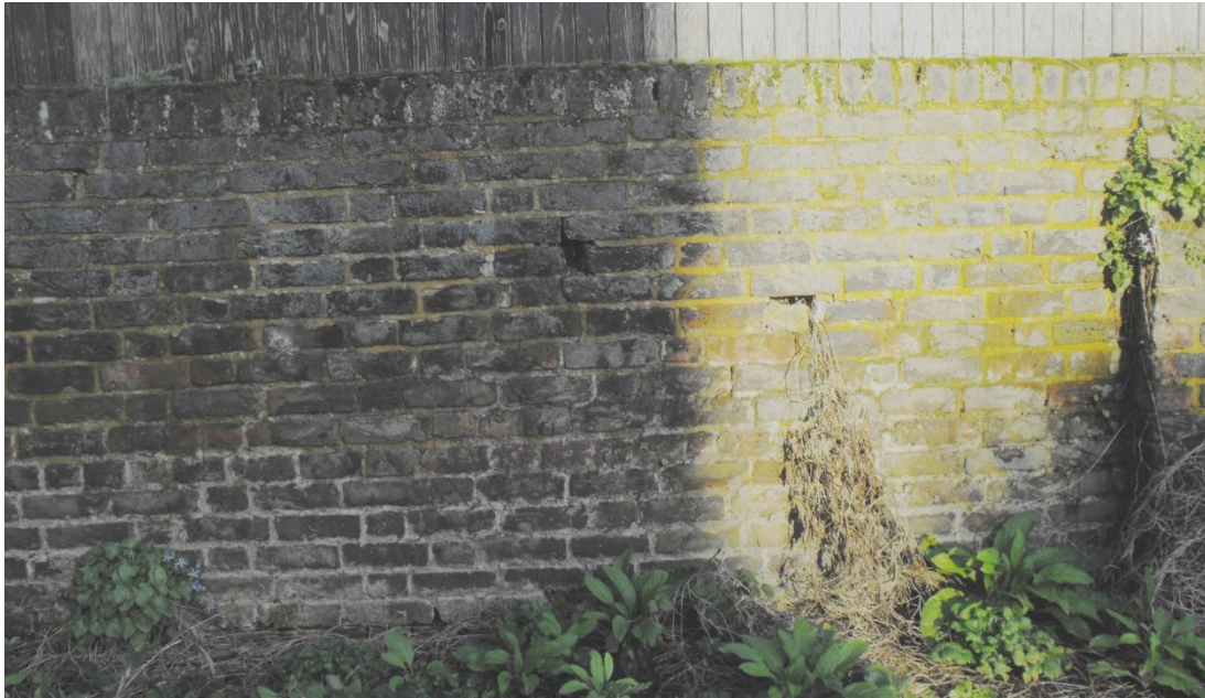
Figure 2: Section B, note missing bricks
