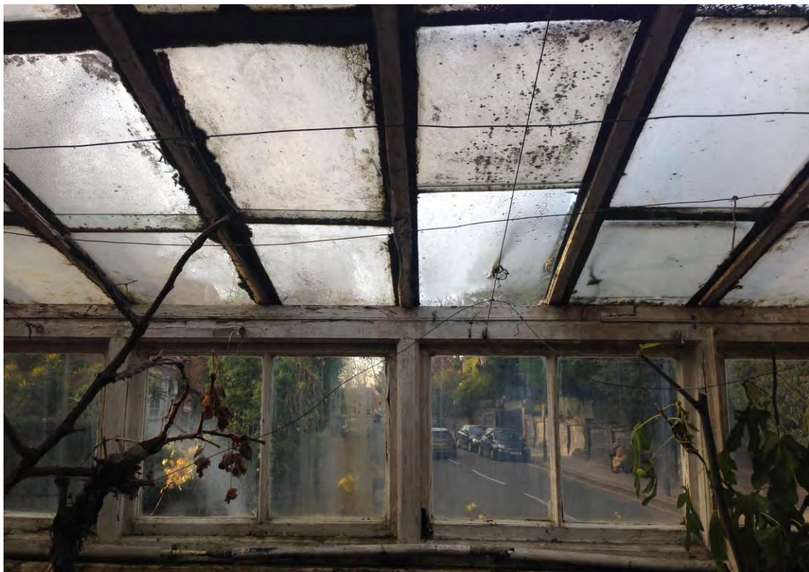
Internal view of orangery which shows the deterioration of the fabric to be renewed / repaired
