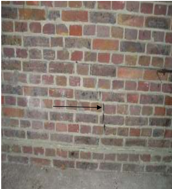
Cracking to left hand flank
