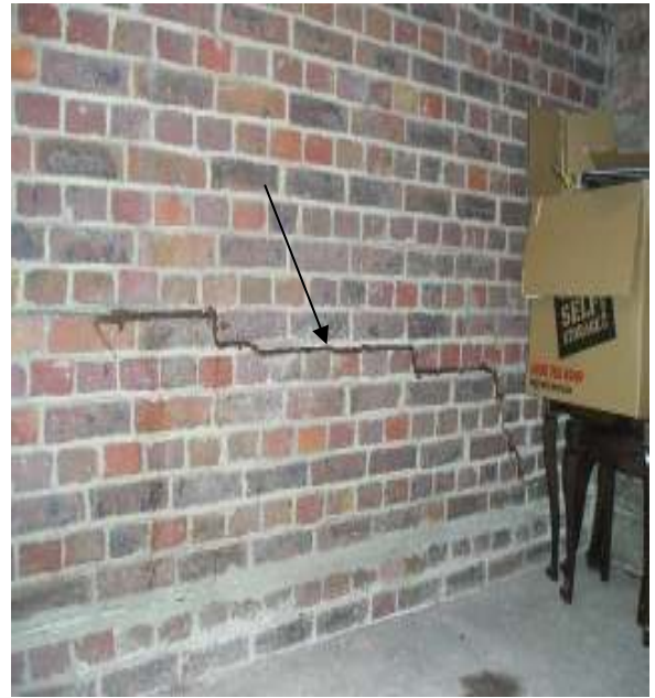
Cracking to left hand flank
