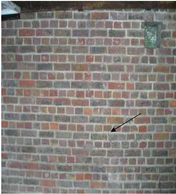
Cracking to left hand flank
