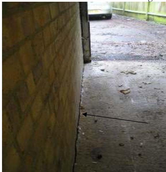
View of movement between slab and right hand party wall
