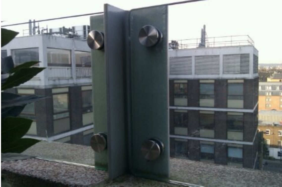
Image 03: existing metal fixings will be retained in situ and will be reused
