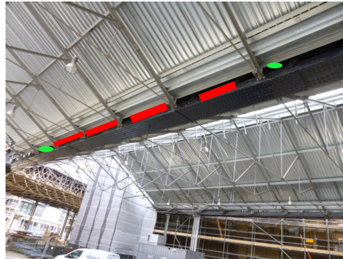
West Handyside Canopy 2 nd North Beam North elevation 4x2 sparrow Terrace + 2 Starling Boxes
