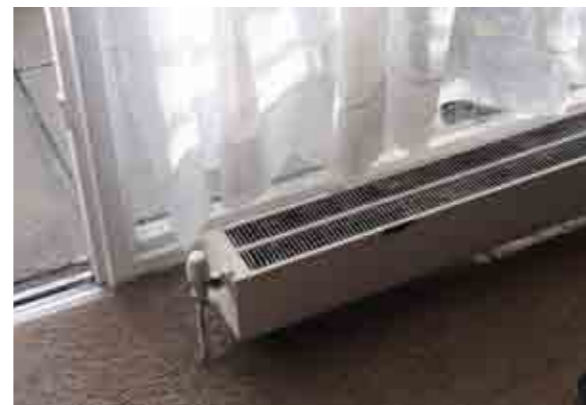
Above: Barrel radiator in front of living room window
