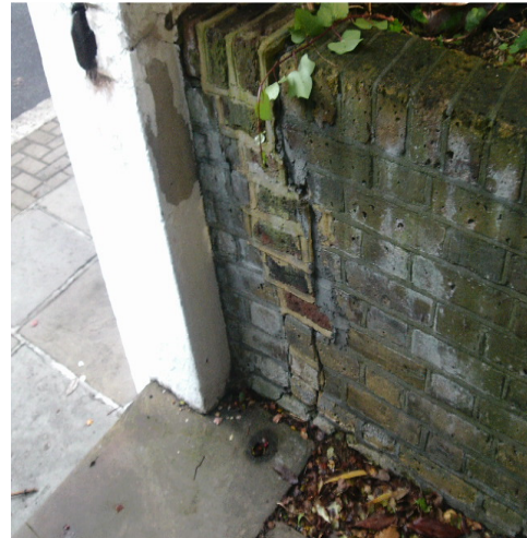
Damage to front garden wall
