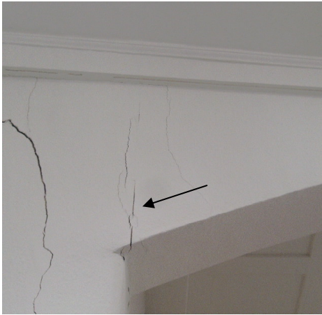
Cracking over arch springing point
