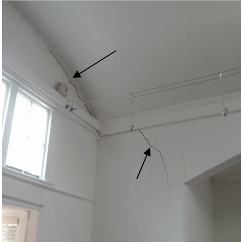
Cracking to front of main room
