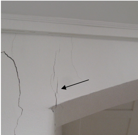
Cracking over arch springing point
