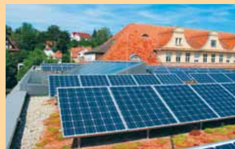
Roof with fully-installed solar energy system.
