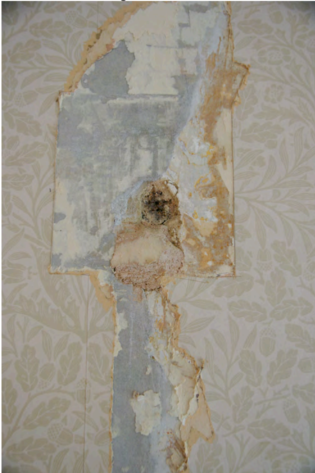
PHOTOGRAPH 3 Wall to 2 nd floor landing – evidence of different material to opening
