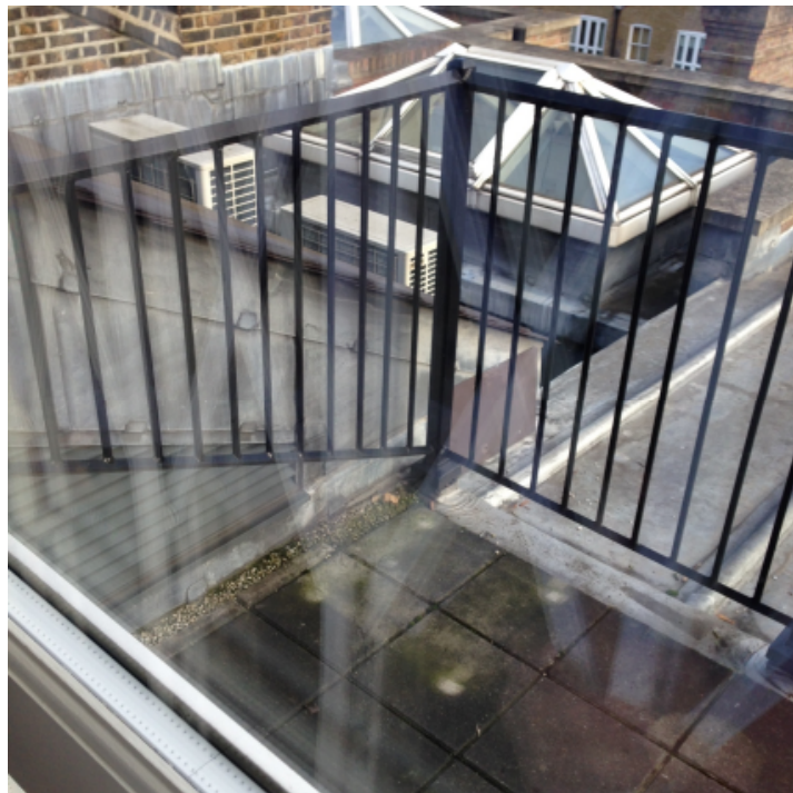
No.2 Existing AC units at 5 th floor level (to right side when viewed from rear)
