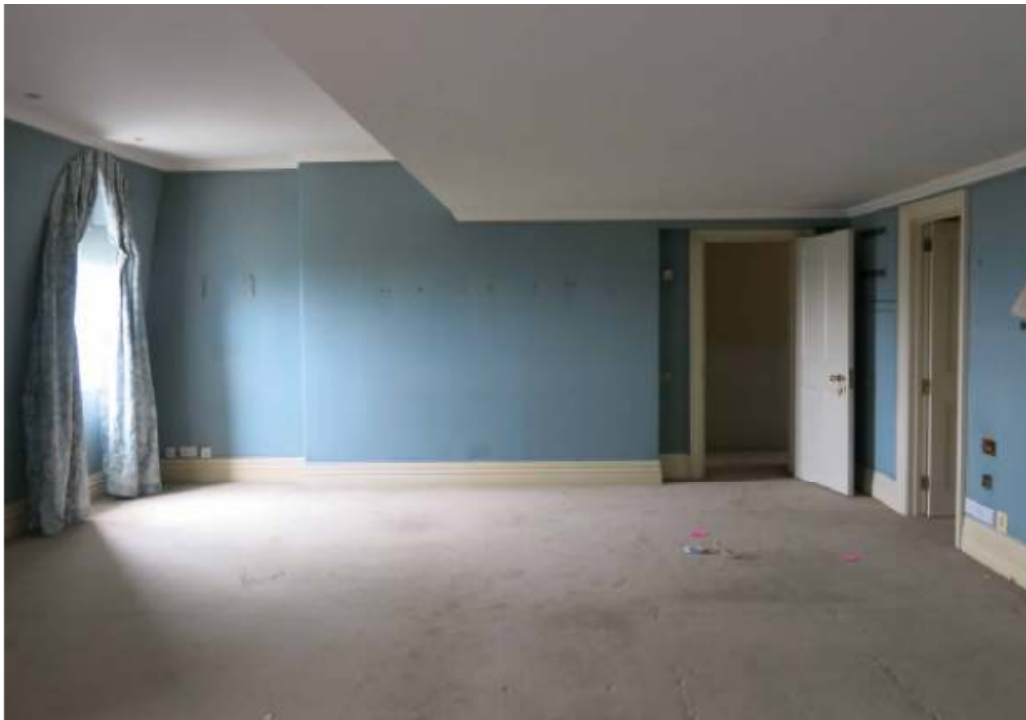
No.8 Master bedroom at 4 th floor where partition walls are to be installed
