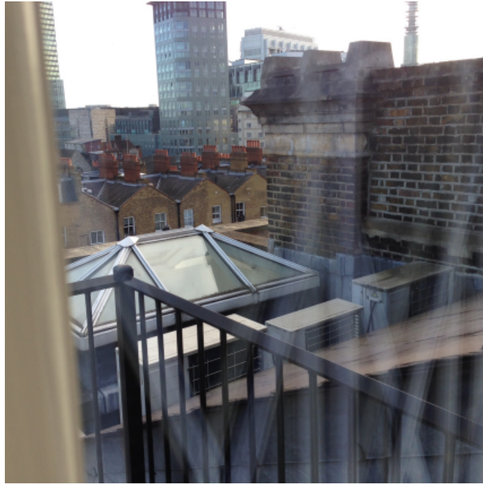
No.3 Existing AC units at 5th floor level (to left side when viewed from rear)
